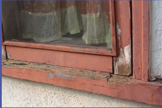
in chipping paint
