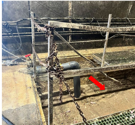
Exhibit 3. The offal wastewater pit on the day of the incident. Arrow indicates where victim likely fell in. Photo courtesy of the employer.
