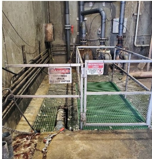
Exhibit 4. The new guardrails and floor grates that were installed after the incident. Photo courtesy of the CA/FACE program.
