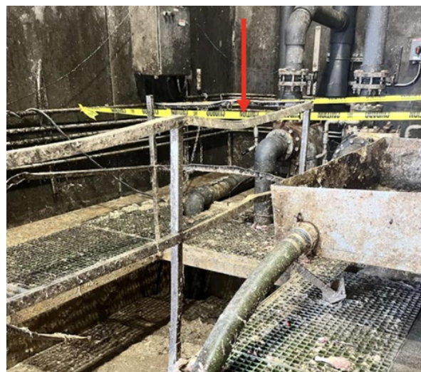
Exhibit 2. One of the damaged guardrails (red arrow) surrounding the offal pit. Photo courtesy of the employer.
