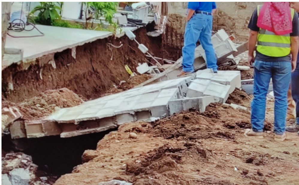
Exhibit 3. The collapsed portion of the wall. Photo courtesy of KTLA 5 News.
